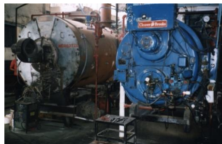
Figure 4-20: Fuel oil operated boilers [74]
